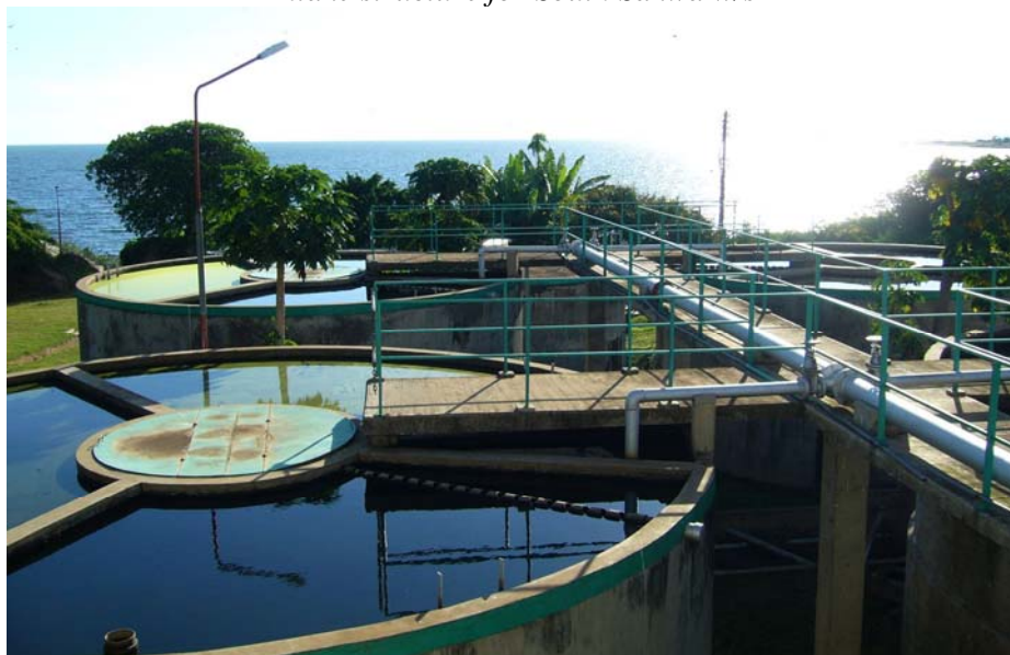
Treatment works at Sakwa
