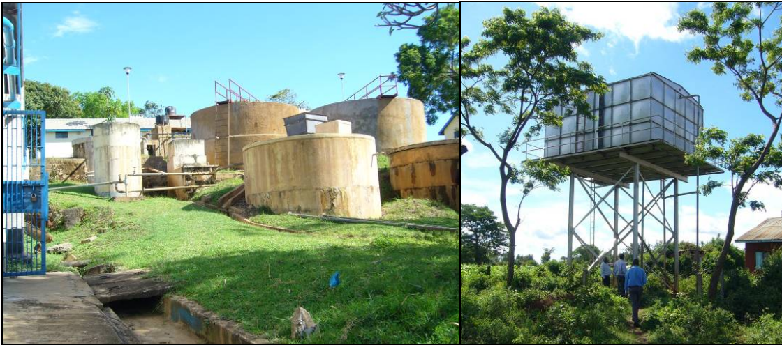
Bondo water supply – Treatment works at Yala River; High-rise storage of 90 m3 in Bondo
