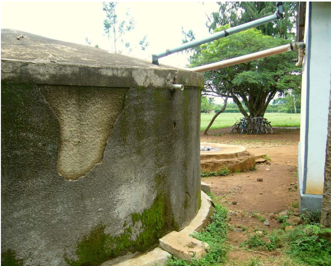
Roof tank for Gobei Secondary School
